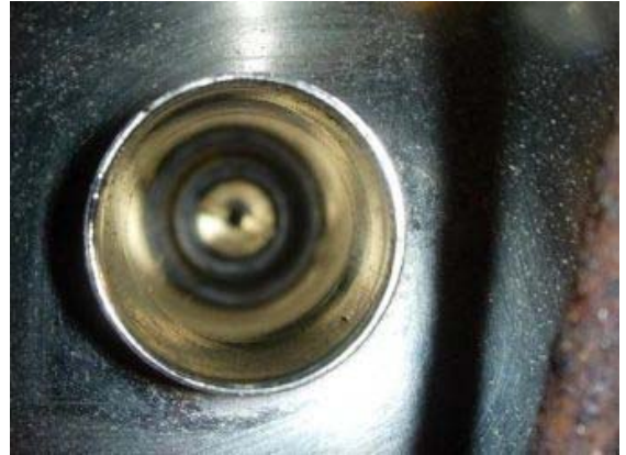
Pic. 50: View into the pump body
